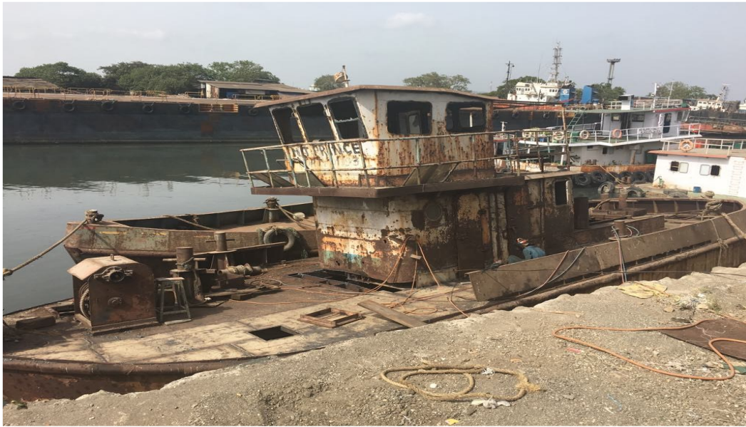
Figure 3, Ship repair work in progress at Darukhana shipbreaking area. © Ayushi Dhawan, 15 May 2018.
